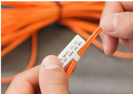
Fibre-Optic Cable Markers
