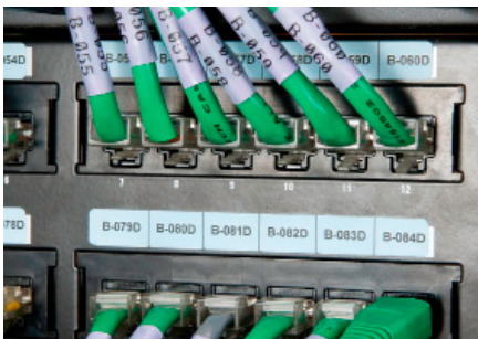
Patch Panel Labels
