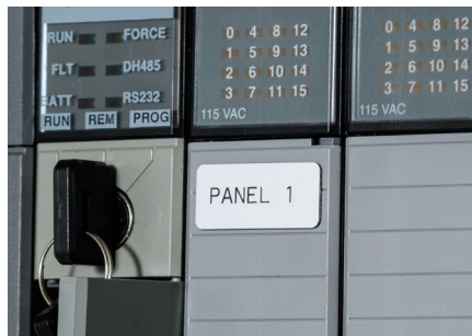
Control Panel Labels
